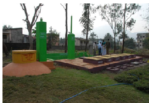
Fig. 9: Side view of the treatment system
